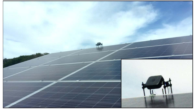
Fig. 10. Experimental setup mounted on top of a roof, with a zoomed detail showing the photograph of the sensor installed on a servomotor and both powered by the battery charger powered by a photovoltaic cell.
